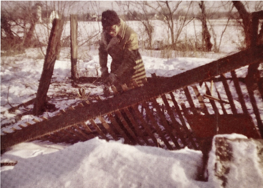
Frank revealed a hitherto unknown capacity for dogged perseverance when he attacked and defeated the endless barbed wire tangle of a long-ago turkey pen, thus clearing needed space for trolley restoration. (TH)
