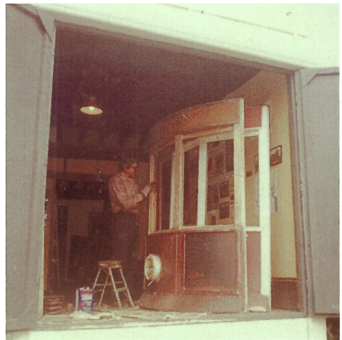
By repurposing a derelict barn on the BR&W railroad property in Ringoes, we provided an all-weather shop, where Frank, seen here, continued preparing one of the complete dash-ends salvaged from the Parsippany car, for eventual installation into 2651. (TH)
