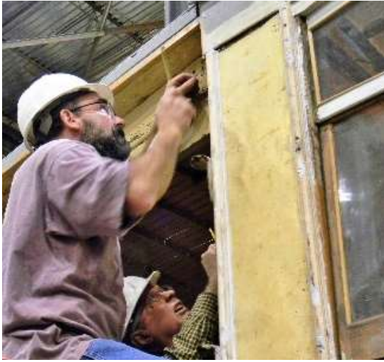
Here Marc is busy replacing missing screws at a corner joint plate.
