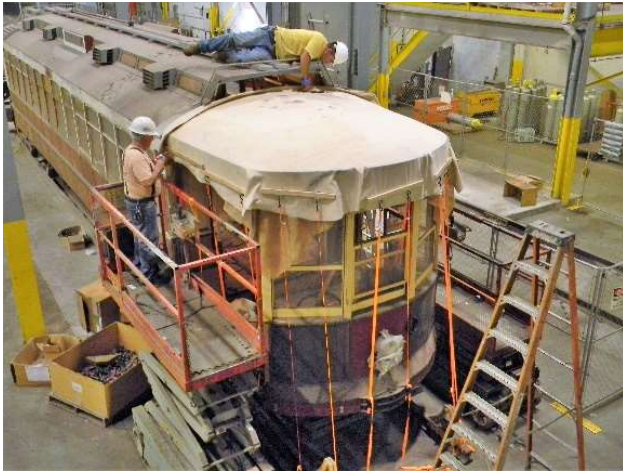
After the canvas had had a week to stretch and settle, the Corps of Restoration begins measuring and predrilling for the many short roofing nails which will permanently hold the canvas in place.
