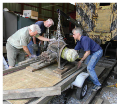
Figure 73: With considerable pushing and pulling, the spare compressor is raised and placed on Bob Hooper's trailer. Photo: DSCN3433
