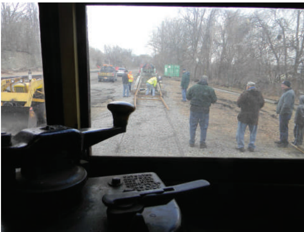
Figure 11: To paraphrase an old aviation cliché, this 100 yards of track will take us 40 miles. Photo: Tony Hall DSCN3195
