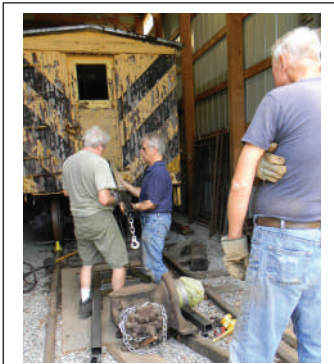
Figure 72: Bob, Hank and Jim secure the chains of Jim's portable lifting hoist to the compressor. Photo: DSCN3426
