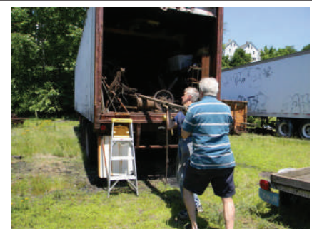
Figure 79: With a final shove the beams are placed into storage. A fork lift would have been helpful. Photo: DSCN3410
