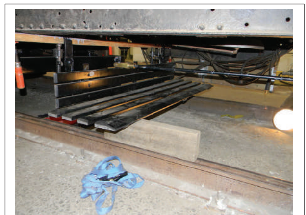
Figure 92: The Basket is successfully clamped into position ready for permanent assembly. Photo: DSCN3400
