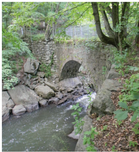
Figure 99: The foot bridge over the river was constructed of hand cut stone quarried on site. Photo: DSCN3415
