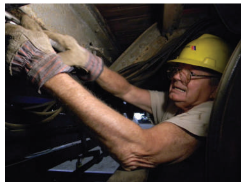
Figure 91: Not John Henry driving steel into a rock tunnel face, just Bob Hooper struggling to get the basket clamped into position under the platform. Photo: DCSN3398
