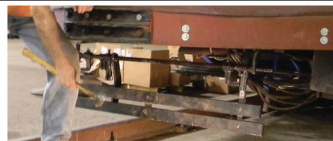
Figure 90: The forward trip gate is hung beneath the extreme front of the platform. Any inward motion of the gate will cause the basket (Fig 92) to drop to the rails Photo: DSCN3392
