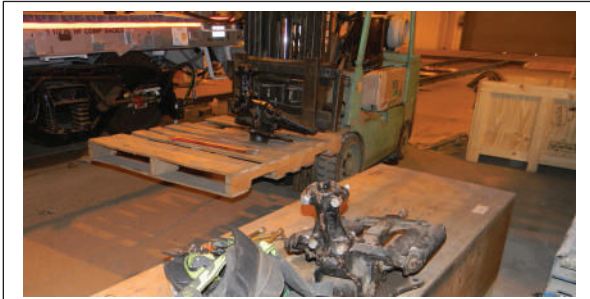
Figure 80: The trolley pole bases are prepared for lifting to the roof. One is in the foreground and one palletized beyond. Photo: DSCN 3272
