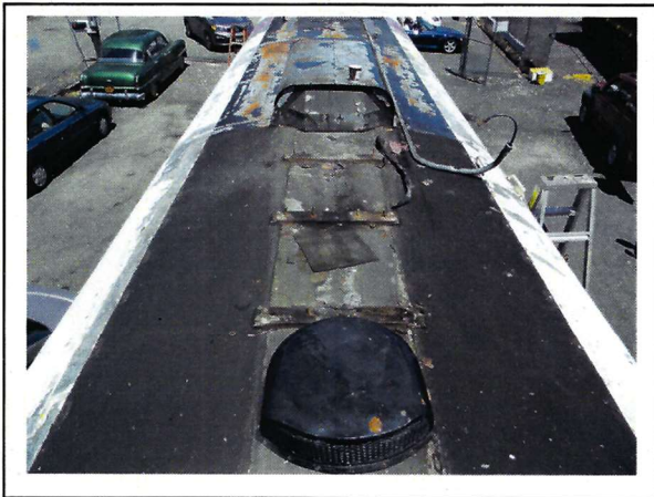
↑With most of the roof fixtures removed, the needed restoration is revealed. The wooden insulating supports showed significant deterioration and will be replaced.
