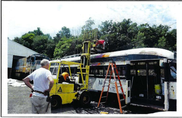
↑Hank Kaminski watches as Jim Tomczyk slides the aftermarket pantograph frame onto the fork lift owned by Star Trak with Nick Ball at the controls.
