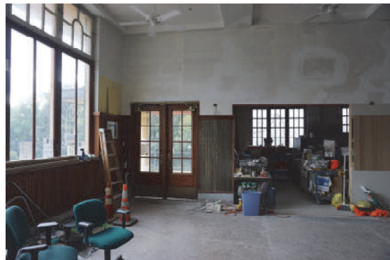
The wall on the Ladies Room side has been partially completed and the windows have been restored.
