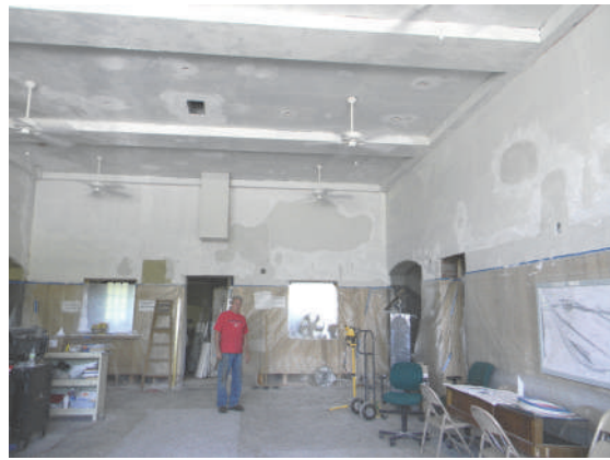
The ceiling in the Main Waiting Room has received its plaster undercoat.
