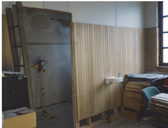
The wall in the Men's room has been completed and the drinking foundation hung.
