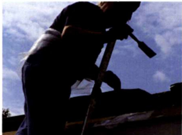
Working without a net, but with an improvised apron, Tony applies roof sealant. 11 Aug 2012, photo by Bob Hooper
