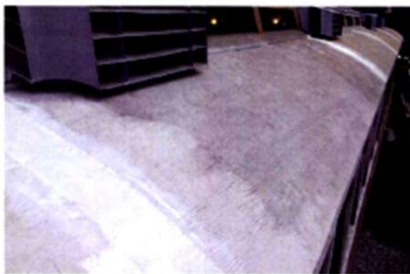
South side lower deck panel joints, having been sealed, await sanding and final coating. Photo by Tony Hall.
