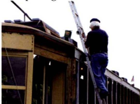
Tony Hall surveys the lower roof deck in preparation for sealing panel joints. 11 August 2012, photo by Bob Hooper
