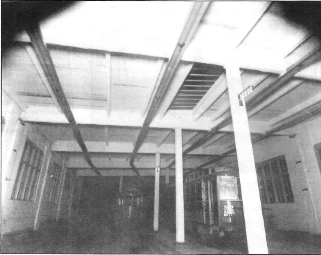
Flashlight view of the interior of South Orange Car House . Based on the wire trough, this view looks south into the shop area from about half way down the first bay.
