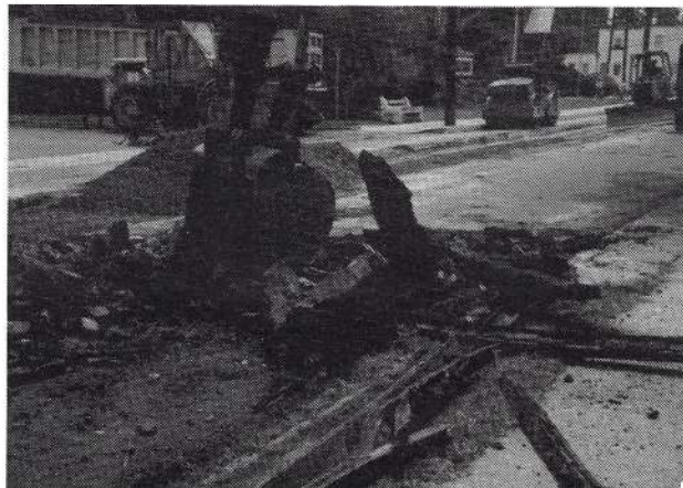
Bill Christian Photo Rail, Ties & Block being removed from Junction Switch - August 15, 1993
