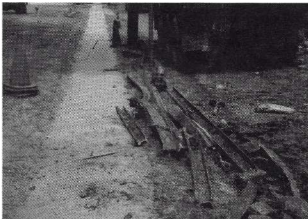
Bill Christian Photo Some of the rail removed from Milltown Junction Switch - August 15, 1993
